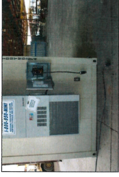
* Showing Power supply line with plug disconnect
