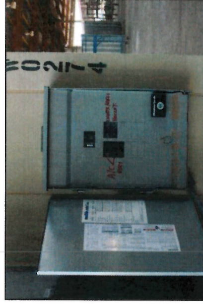
Electrical Panel showing Main Disconnect and Circuit Breakers
