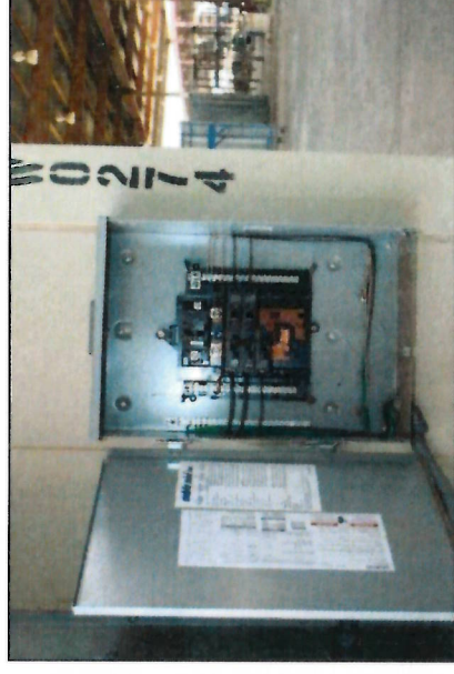
Cover Removed, where electrician will make power supply connections
