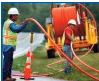
Broadband/Fiber Optic Cabling
