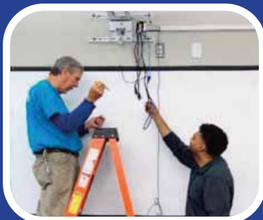
Mary Ellen Stempfle University Center Smart Technology Installation
